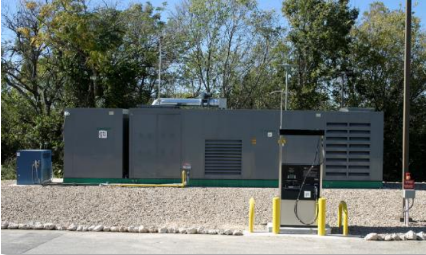
UT-CEM / GTI Hydrogen Fueling Station – first in Texas
