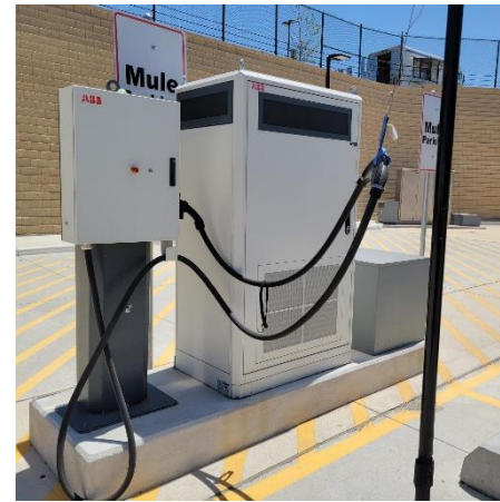
LSEV Charging Station
