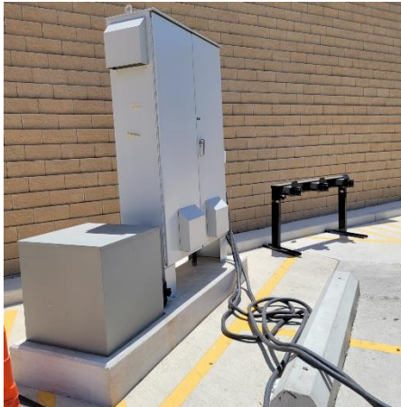
Orange EV Charging Station
